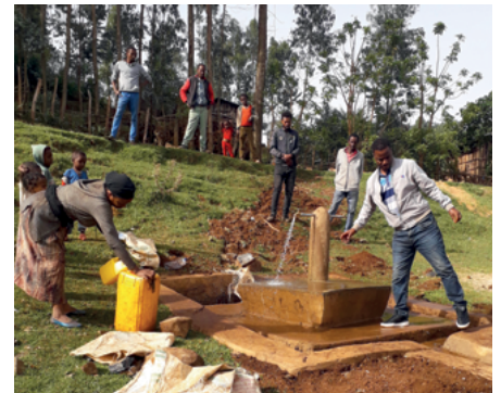
The new water point in Ambacho
